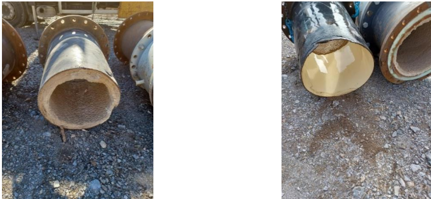
Figure 8: Before and after the application of sonic pulses on a 600mm pipe with 9cm thick calcium carbonate deposits.
